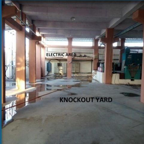
Knockout Yard with Electric Panal Board View
